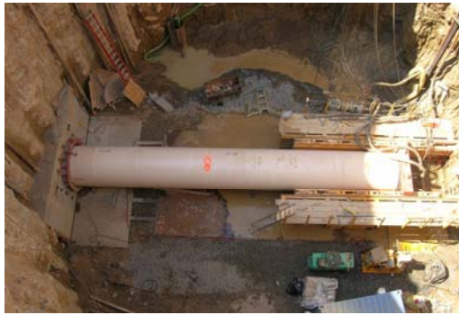
Intake installation from wet well
